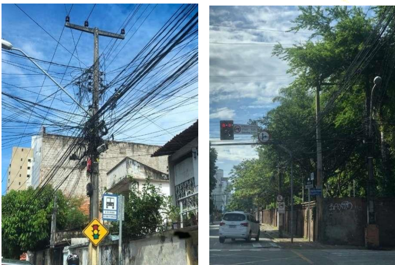
Figures 05 and 06 - Entanglements of wires in electric pole
